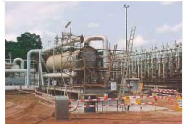
Gathering station heat exchangers in an African oil field presented a big cleaning challenge for AIMM Technologies of LaMarque, Texas.
